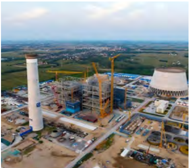
Yuncheng 630° C national power demonstration project
