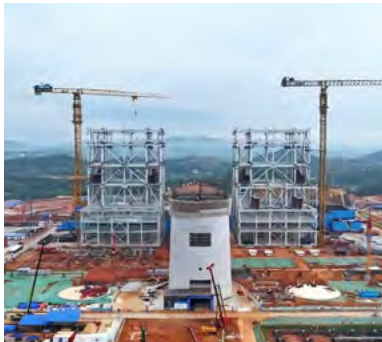
Zhuzhou 2×1 GW capacity expansion and upgrade project
